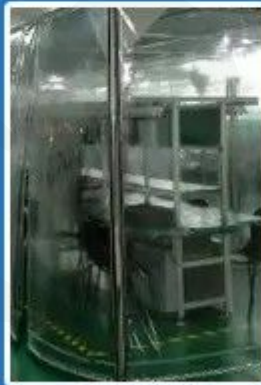
Clean laminar flow zone
