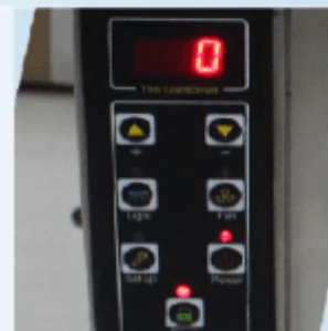
Control panel Working state of digital window LCD
