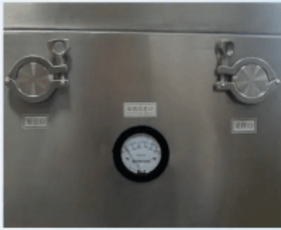
Differential pressure gauge
